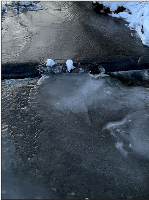
Slush and ice below Bridge 1 on December 21 at 7:40 AM Temperature: air, -13°, water, +0.2°
